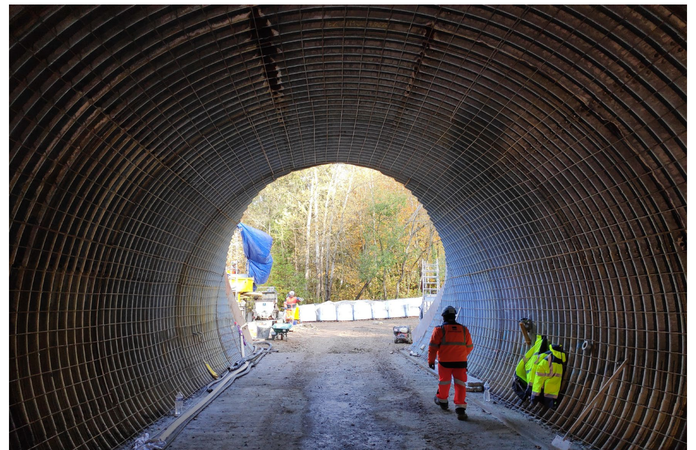
Buse de Sevenans, France, 2020 - Freyssinet
