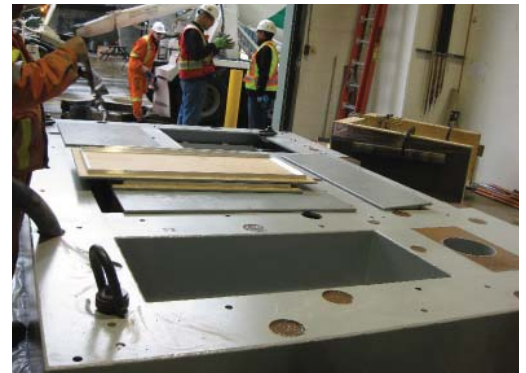
UltraSeries™ Heavyweight filled the steel form of the North hot cell roof uniformly and without incident.
