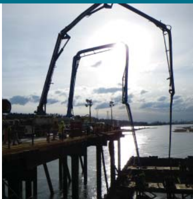
Left: Two 52 meter pumps were used to pour Agilia® Architectural into the cofferdams. A 36 meter concrete pump and a box remixer were used to feed one of the larger pumps.
