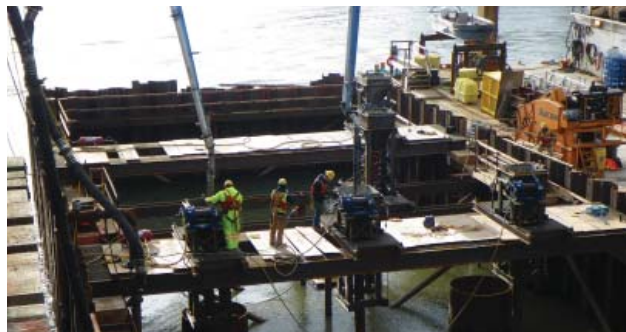
Agilia® Architectural was used to create tremie concrete plugs for 5 cofferdams across the Fraser River. It's high level of flow, SCC properties, and paste retention made it well suited for an underwater pour.
