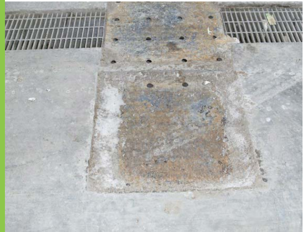
After 3 years of being in operation the Extensia® Slab at the Cold Lake Waste Transfer Unit exhibits minimal cracking.
