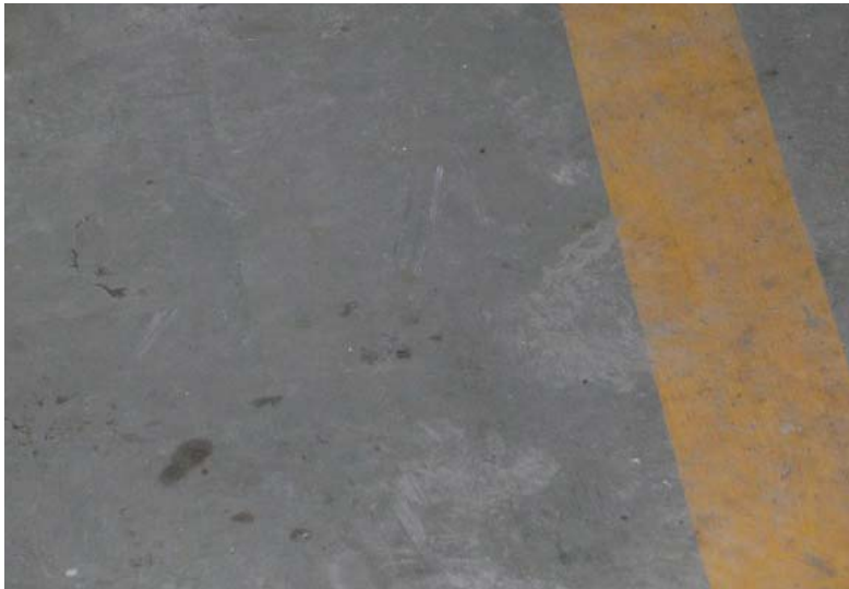
A close-up of the 3 year-old Extensia® concrete pad at the Cold Lake Waste
